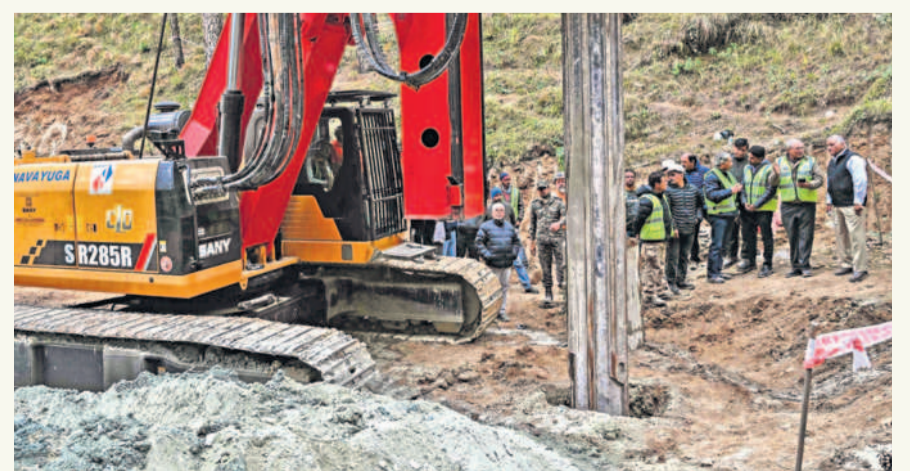
The earth-boring machine deployed to drill a vertical hole into the collapsed tunnel. — Photo: AFP
