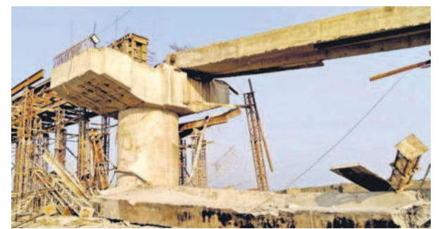
The part of under-construction bridge which collapsed in Bulandshahr on Saturday. — Photo: PTI
