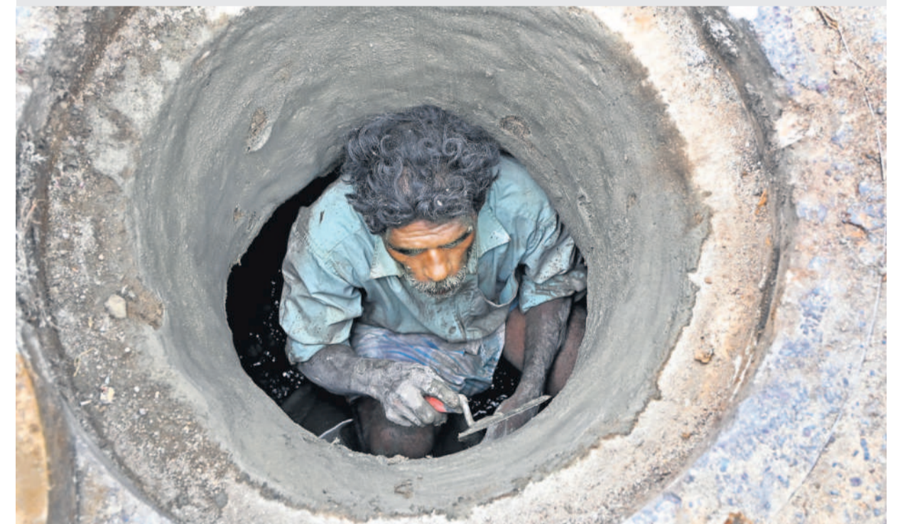
A worker plastering the inside of a manhole with cement on a busy road in Hyderabad on Wednesday. — Photo: Surya Sridhar
