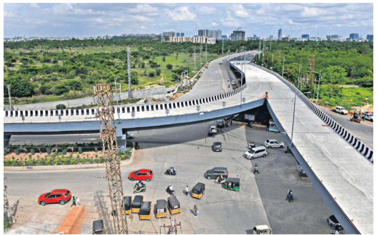
The flyover at Gopanpally was expected to be inaugurated after LS polls in June once the poll code was lifted. — Photo:Anand Dharmana
