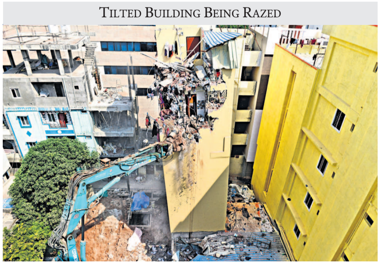
GHMC started demolishing a four-storey building, which tilted to one side, in Gachibowli on Wednesday. The building started to tilt on Tuesday after earth in the adjacent plot was excavated to build a cellar, disturbing its foundation. — Photo: Anand Dharamana (REPORT PAGE 3)
