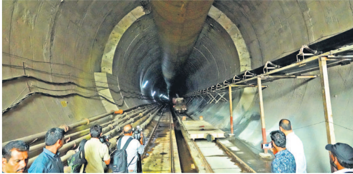
The under construction stretch in the tunnel of Srisailem Left Bank Canal (SLBC) project where a section of roof collapsed, in Nagarkurnool district on Saturday.
