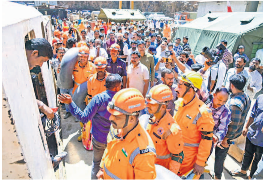
Rescue operations on at the SLBC tunnel project site in Nagarkurnool on Sunday. — Photo:PTI
