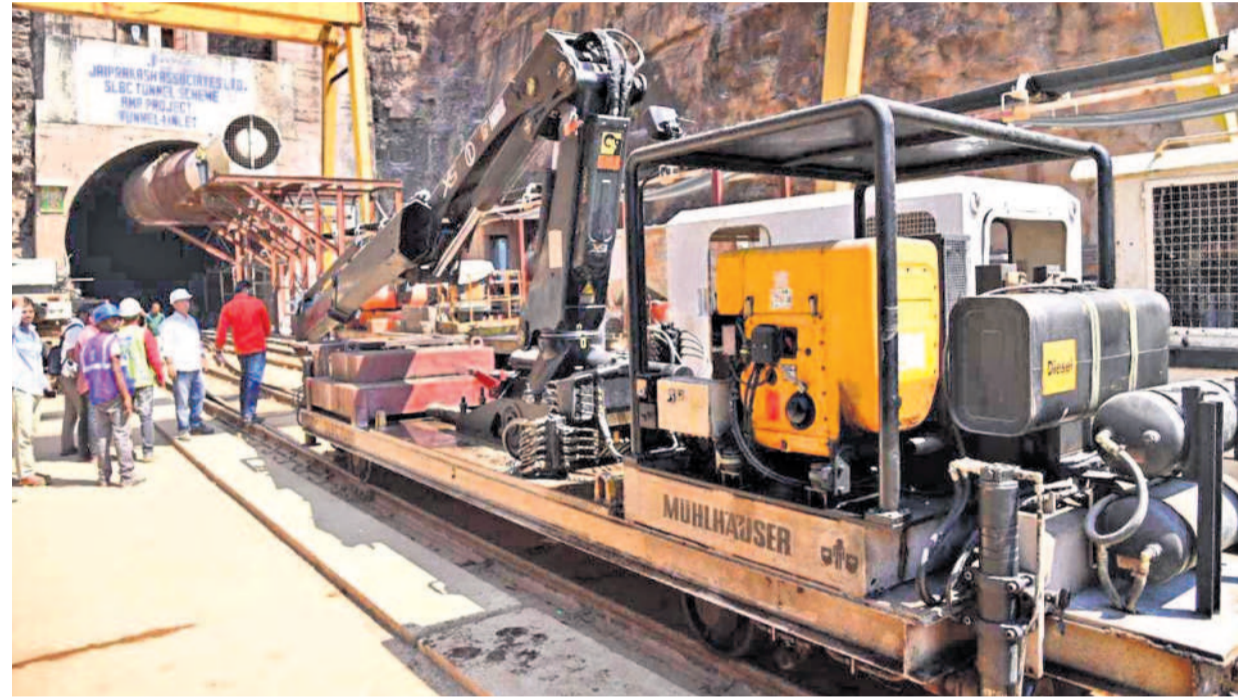
The SLBC project site where a portion of the tunnel collapsed, in Nagarkurnool district on Tuesday. — Photo:PTI
