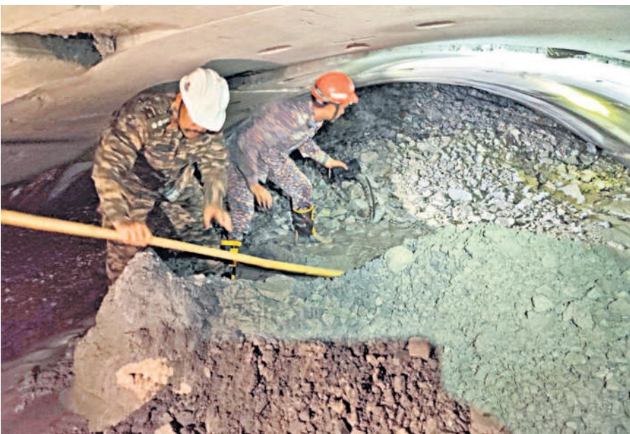
Experts involved in the rescue operation suspect that the workers might be trapped beneath the damaged tunnel boring machine.
