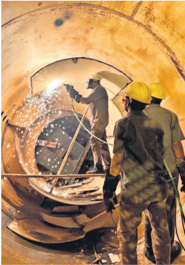
Rescue operations under way at the Srisaillam Left Bank Canal tunnel collapse site in Nagarkurnool on Saturday.
