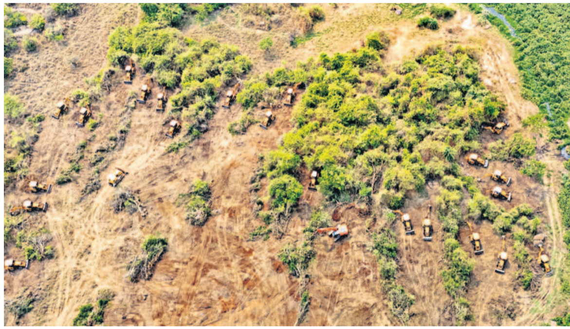
Excavators deployed to clear the forested land at Kancha Gachibowli on Monday.
